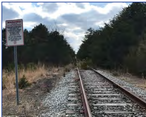
Current condition of former Reading Company's Cape May Railroad Tracks near Woodbine Junction
